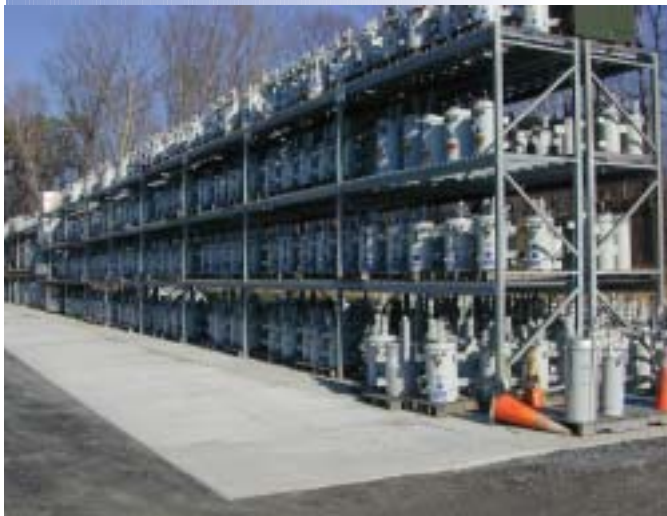
Below: This storage rack contains dozens of transformers of all sizes.
