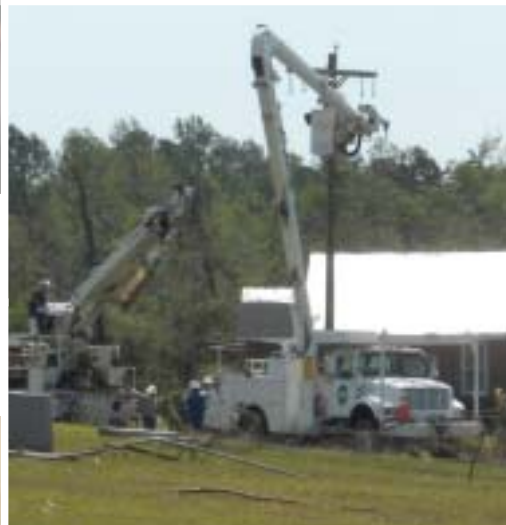
REMC crews traveled to various states to aid in restoring power after storms. Here, crews repair tornado damage at a church in Eutaw, Ala.
